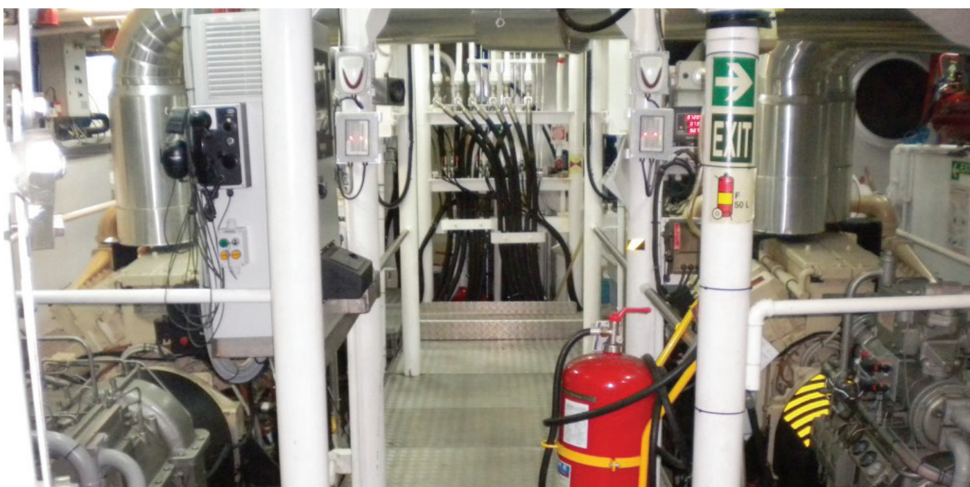
Filomena's Engine room
